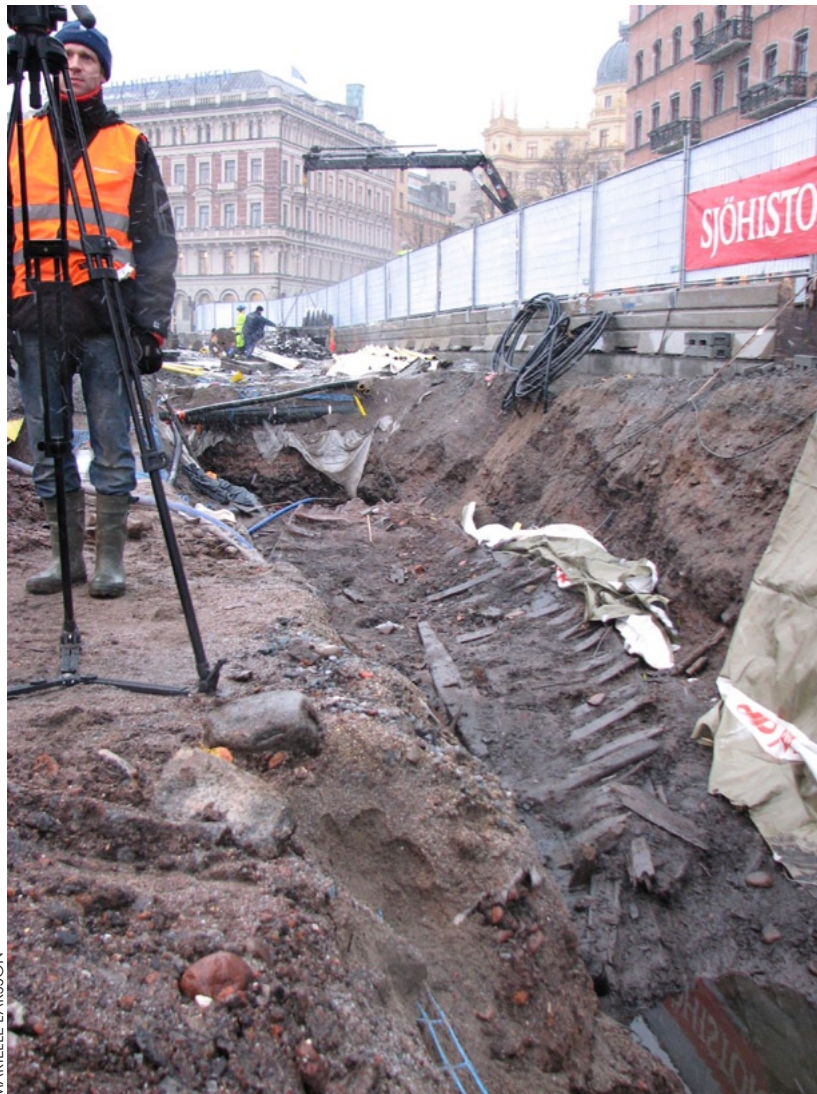
The Maritime Museum in Stockholm is excavating an area in the city center. In front of the Grand Hotel, the remains of a wreck that was sown together was found
