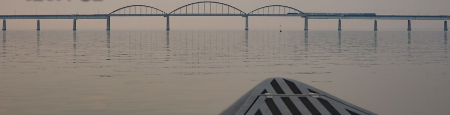
Storstrømmen and the bridge from 1937, which is corroding and going to be replaced with a new one.
