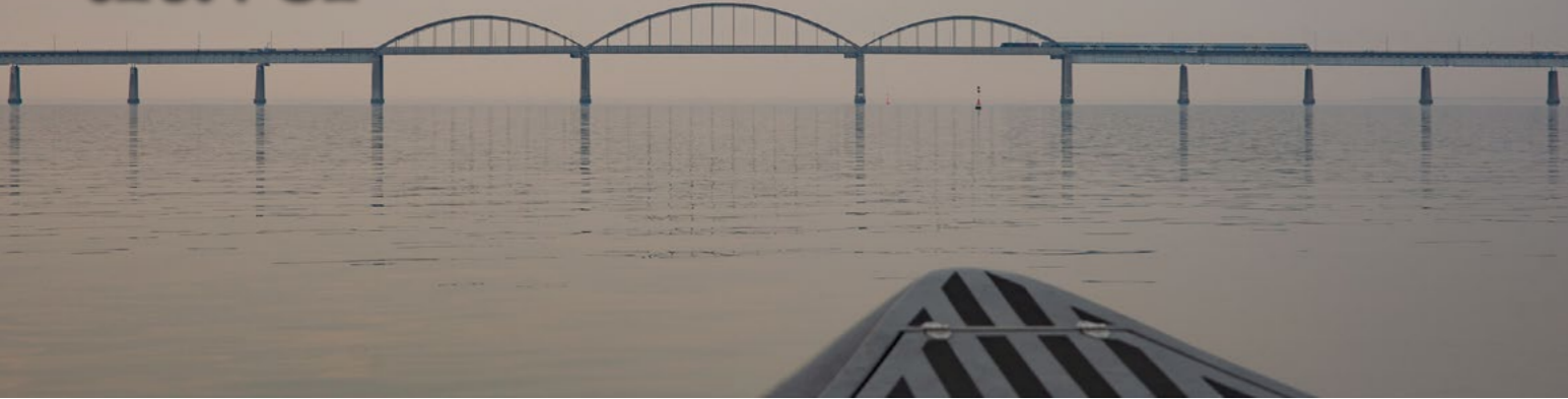
Storstrømmen and the bridge from 1937, which is corroding and going to be replaced with a new one.
