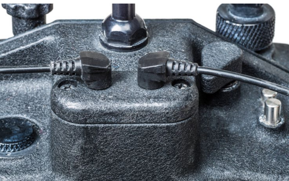
Fiber optic cables attached to a housing
